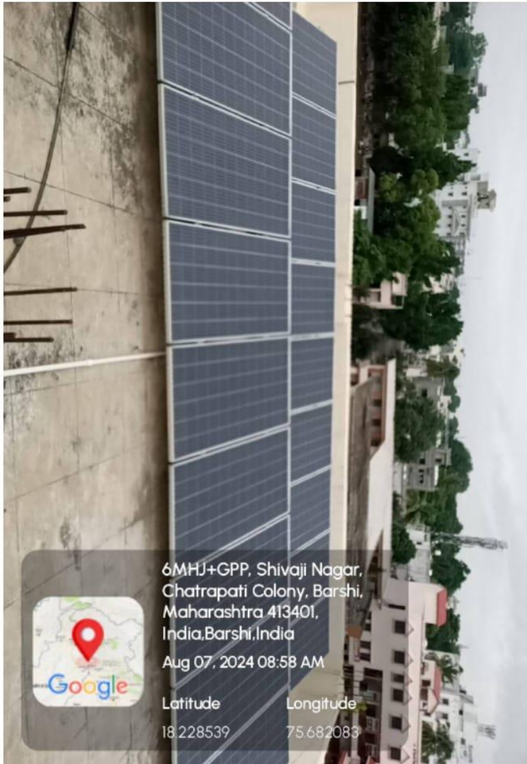
Solar Panels on Library Building
