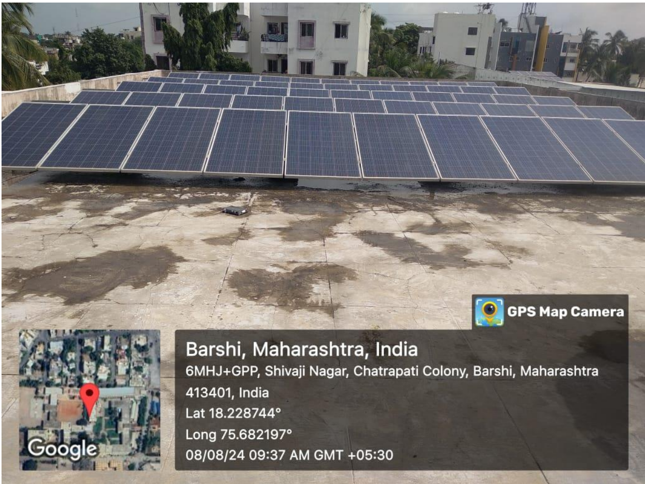
Solar Panels on Library Building
